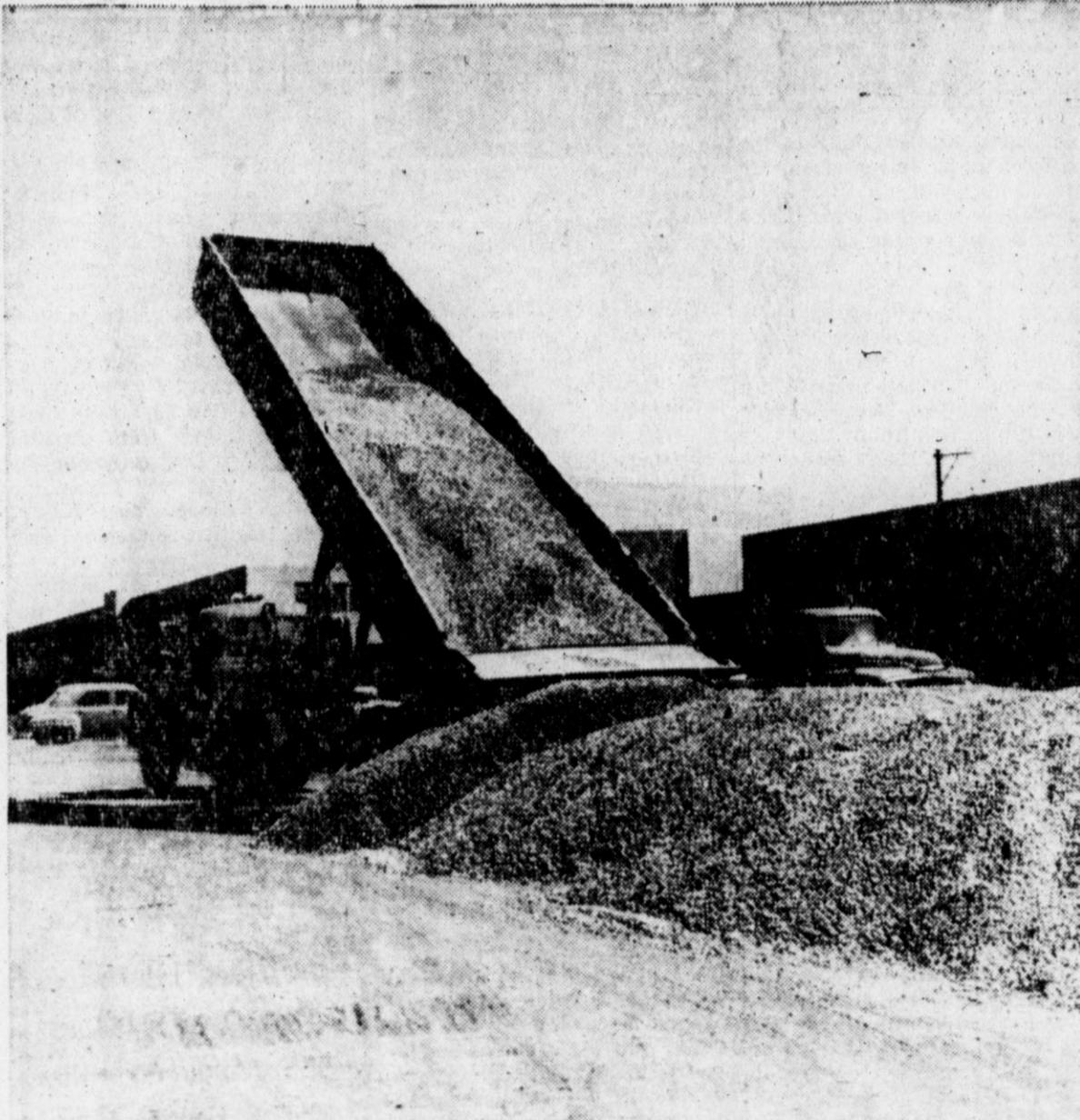
GRAVEL for use in paving projects at Aik-near the high school. A truck is shown near Elementary and Hereford High School dumping a load of gravel. (Staff Photo) parking areas was stock piled last week
