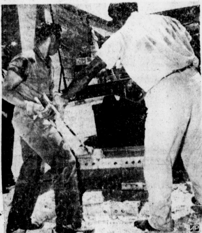
WORKMAN ROBERT McGEE, left, and Kinley Cestine are shown lifting part of the brick wall which fell and buried Gloria Rivera, 13, of Houston at the J. L. McReynolds Junior High School. Three teen-age boys admitted accidentally pushing over the wall as a student prank. They said they were trying to rock a school bus backed up near the wall by bracing themselves against the wall and pushing against the rear of the bus. (AP Wirephoto)
