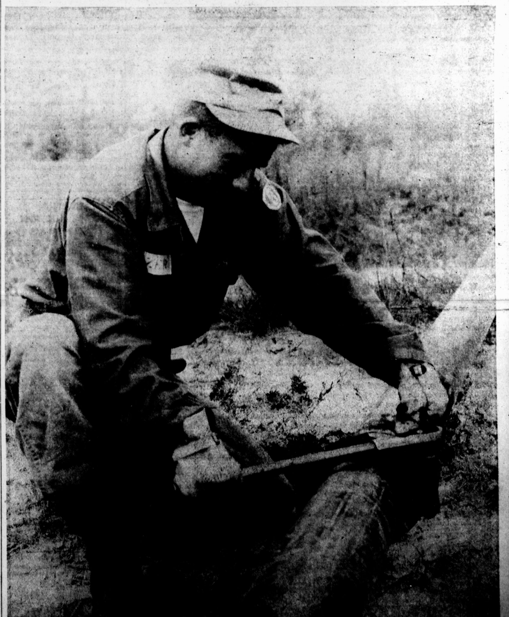
SPECIALIST EUGENE M. ZINSER of Hereford is shown tightening the coupling on a six-inch pipeline being laid by the 700th Engineer Pipeline Co. now in summer campment at Fort Polk, La. The 700th Engineers has a platoon in Hereford, under command of Lt. James Alston.
