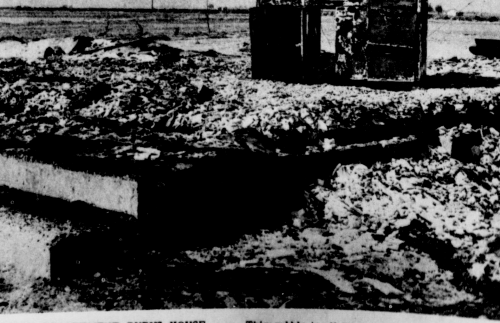
FIRE DEPARTMENT BURNS HOUSE . . . This rubble is all that remains of a house belonging to Gary Miller that was burned down last week on the request of the owner. Supervising the burning of old, delapidated houses and buildings is another service performed by the Bailey County Volunteer Fire Department.
