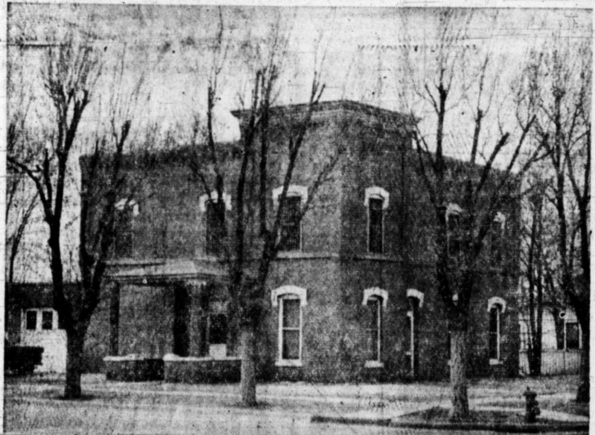
The present Deaf Smith County Jail has bulged of the structure. Cracks are prominent in the walls on the north, south, east and west sides.
