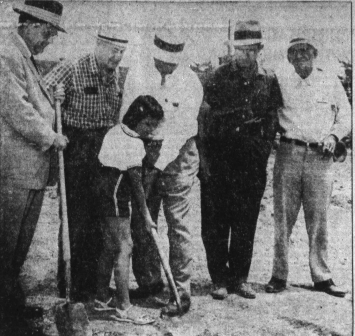
GROUND BREAKING CEREMONIES —Sue Ellen Douglas, 7, took delight this week in turning the first shovel of dirt to begin construction of the new $60,000 Hereford State Bank building at Third and Sampson. She is the daughter of Townsend Douglas, left, bank president. Present for the occasion were Bill Lenderman, R. G. Peeler, a stockholder who gave Susie an assist, Robert Thompson, contractor, and Walter N. Hodges, bank director.
