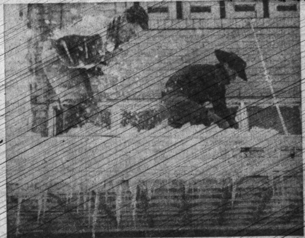
AND THE SNOW FLIES —Don Jackson and Garth Smith get busy getting snow off the top of the Western Auto store after the roof of at least two local stores caved in due to the weight of the 27 inch deep snow. (Staff Photo)
