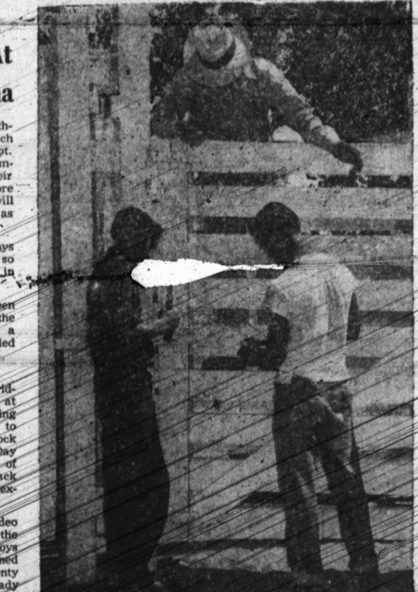
READY FOR RIDES —Boys Ranch rodeo facilities have been completely rebuilt this year. Putting final touches to the new chutes has kept the boys busy getting ready for the annual event, Sept. 2-3.
