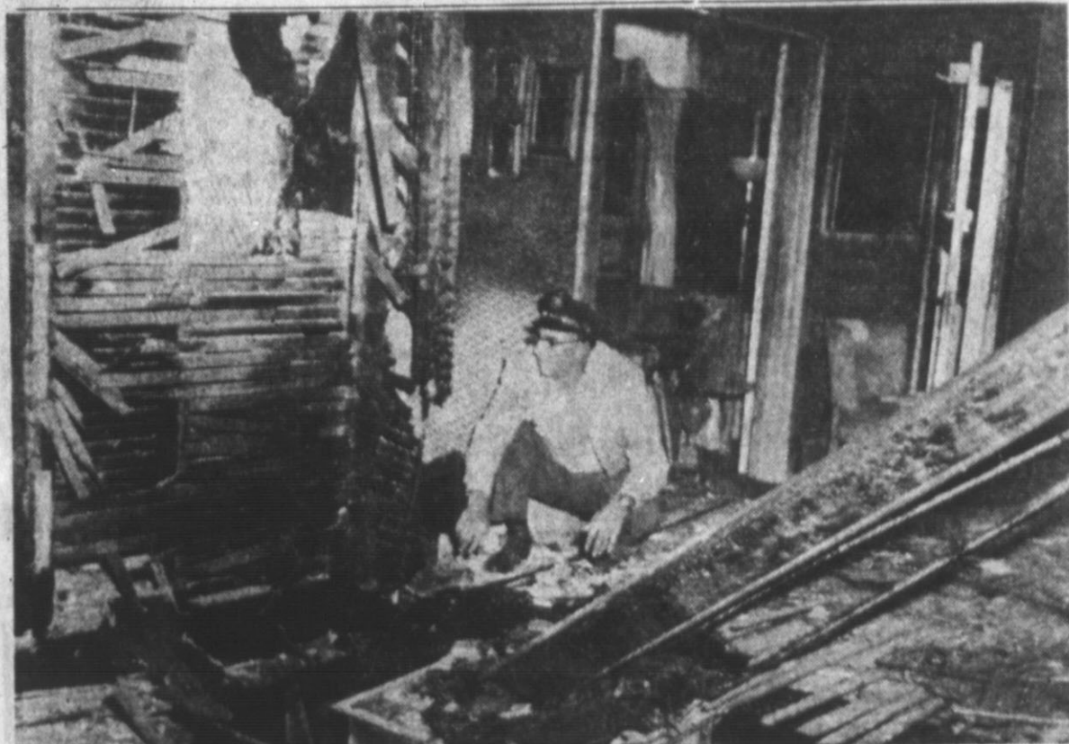
HERE'S WHERE IT STARTED — Clay Angelo, fire warden, points to the floor furnace in the Bob Cummings' home, 504 West Third, where fire which almost totally destroyed the interior of the house, is believed to have started. Damage was estimated at $5,000. The Cummings were out of town when the fire occurred. (Staff Photo)
