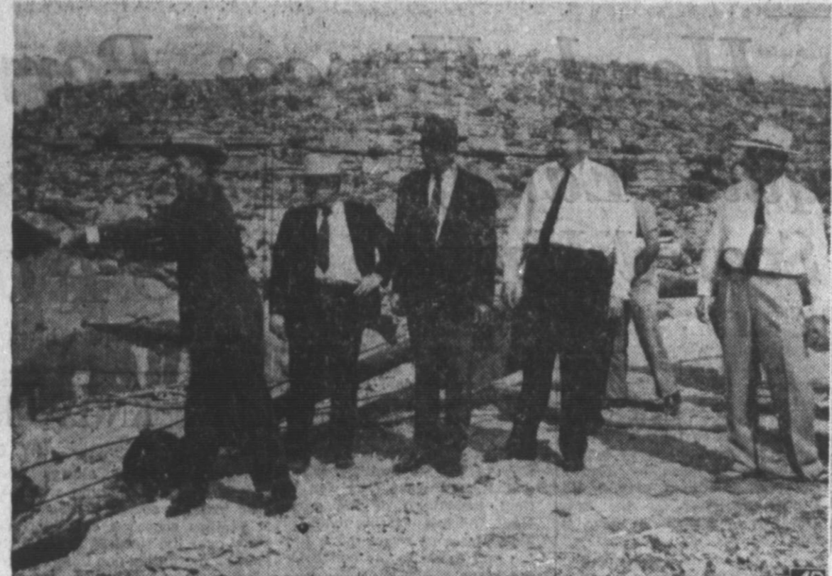
PECOS RIVER BRIDGE STARTED — Turning a shovelful of dirt and rock marking the start of construction of the new highway bridge across the Pecos River north of Del Rio is E. H. Thornton, Jr., chairman of the State Highway Commission. Looking on are, left to right: Highway Commissioner Marshall Formby; Jack Rhone of Del Rio; Herb Petry, member of Highway Commission; and John L. Dodson, Jr. The new bridge will span the canyon from side to side and will be over 300 feet high. (AP Photo)
