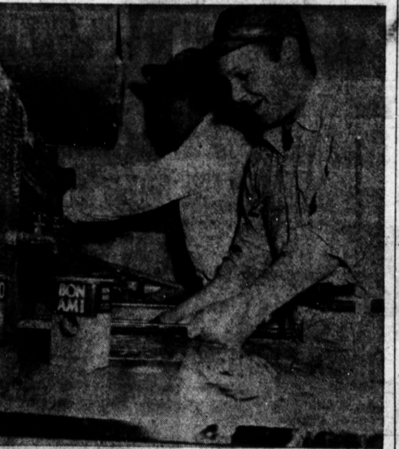
SOME OF THE FINISHING touches for the Kitchen-Clubroom included scrubbing down the last few parts of the range and putting plastic tile around the sink. George Loerwald was handling the first job, while Bill Brodie carefully fitted the tile into place. (Staff Photo)
