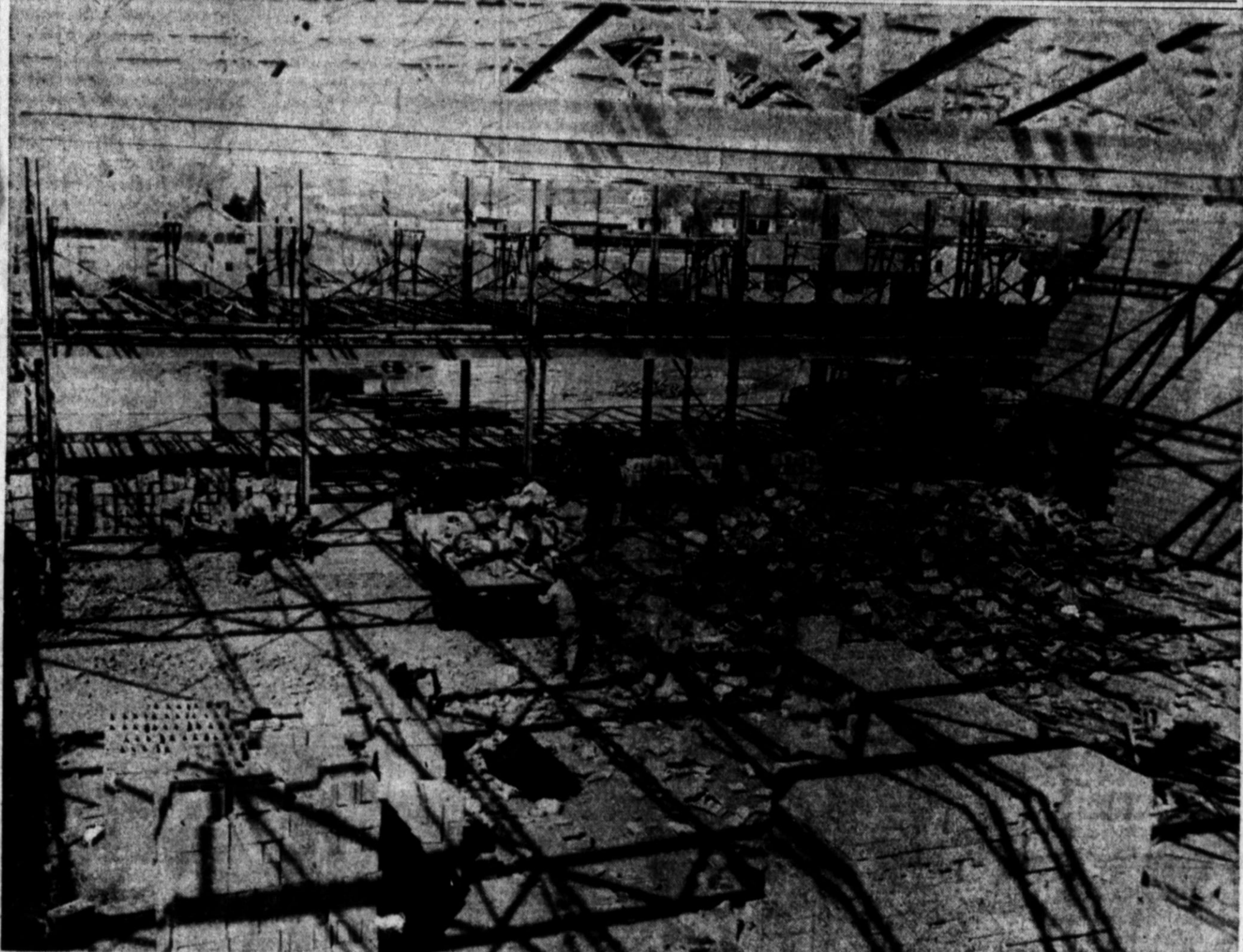
ONLY 15 MINUTES before the west wall of the gymnasium in the new high school building fell inward because of pressure from the high winds Thursday morning, workmen were called off that part of the building because the wind was blowing too hard for them to work. The wall was built of Haydite block, and had been faced for eight feet up on the inside with
