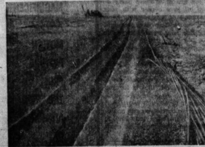
Longer gas pipelines can be installed at a lower cost with Carlson plastic gas pipe. Hundreds of miles of trouble-free pipelines have been installed in Texas High Plains area.
