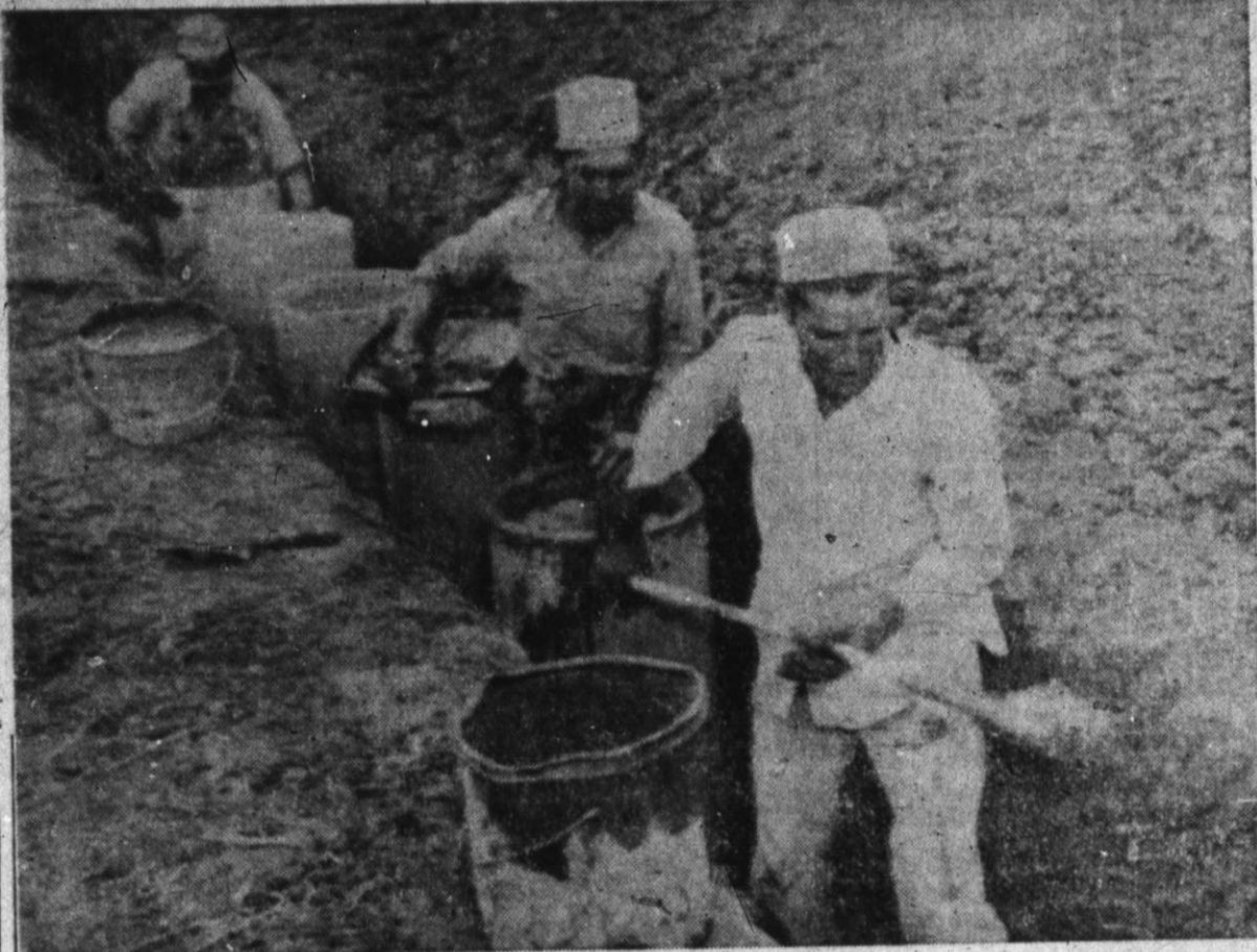
HERE IS THE "assembly line" used in laying underground irrigation pipe on the H. A. Wells farm at Friona. The man in front is the most important member of the crew. He is called the "Brusher" and seals
