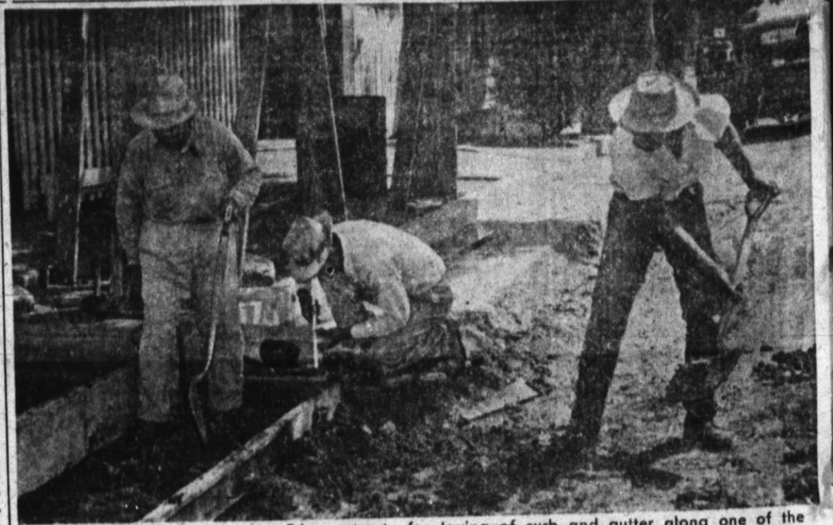
WORKMEN ARE preparing Friona streets for laying of curb and gutter along one of the many blocks slated for improvement there this summer. This scene is typical in Friona these days as the town is quiet with building and improvement activity.—Brand Staff Photo.
