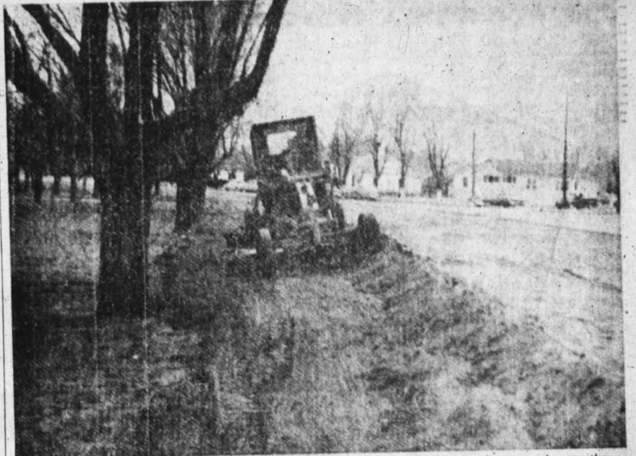
WORK ON LAKE park is progressing this week as the grader shown above works on the terracing at the park's main street boundary. Shrub and tree removal has also gotten into high gear for the park's renovation program.—Staff Photo.
