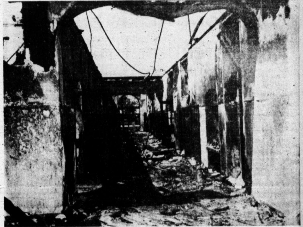
THE FIRE-GUTTED interior of the Friona high school is slowly showing signs of clearing as clean-up operations get underway. No plans have been announced as yet by the school officials for rebuilding the structure, which burned the morning of May 16 with a resulting loss of over $100,000. This picture shows the destruction looking up the north hall of the Friona school. Brand Staff Photo.
