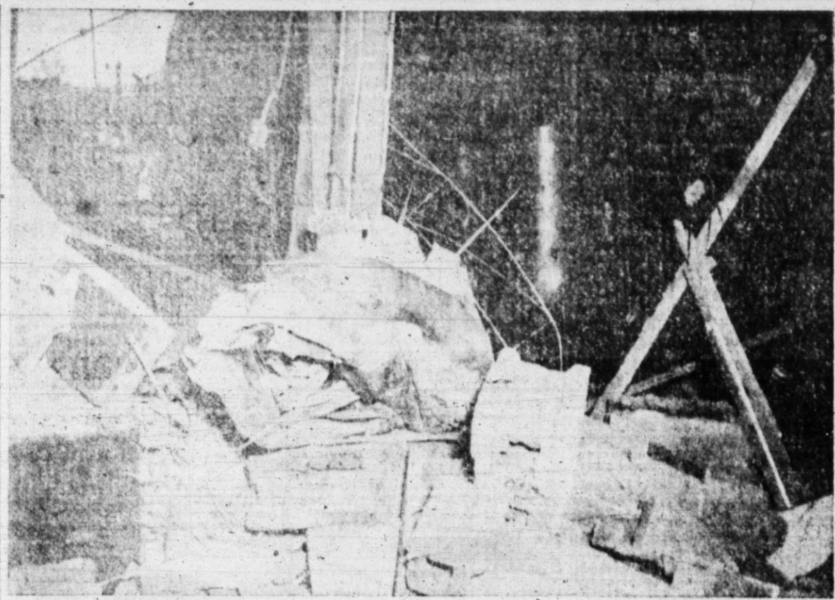
THE JACKET of the hot water heater that caused the blast Monday at the Park Avenue Village shopping center is shown in the above picture after it had pierced the wall after curling off the insides of the heater. The picture shows part of the 50-foot hole torn in the rear of the newly-constructed building.—Brand Staff Photo.
