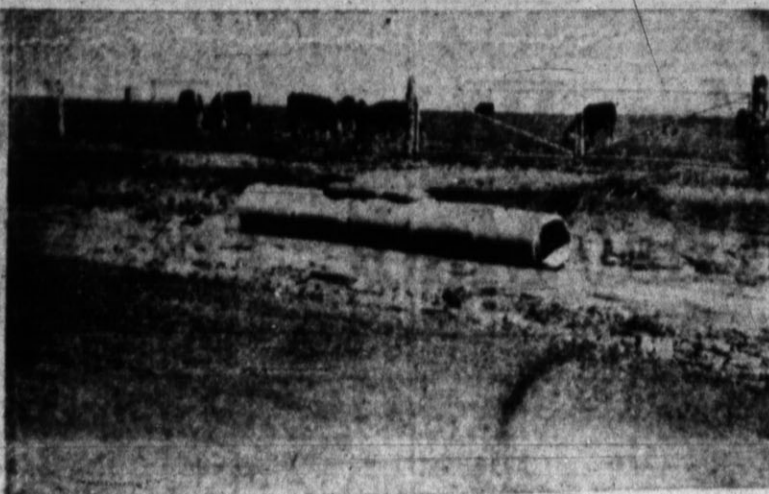
WASHED OUT CULVERT —Excessive rain washed out this culvert along with considerable other damage which set the highway completion date back about two weeks and cost about $5,000 extra.
