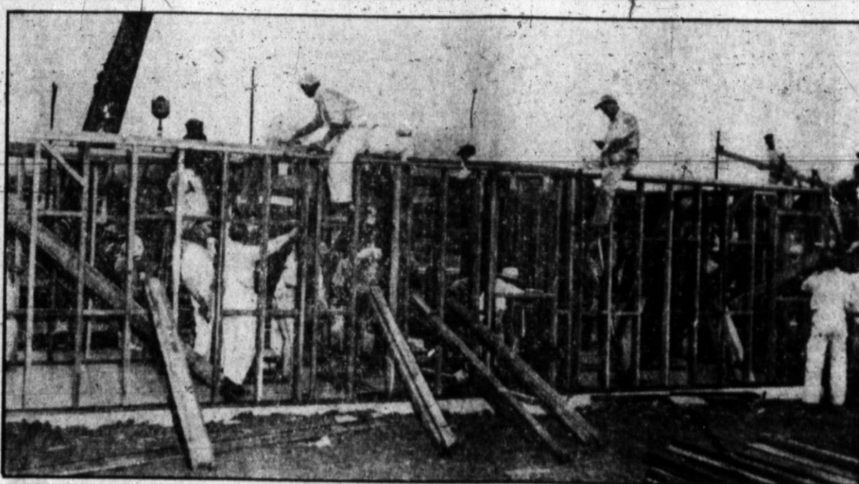
HOME WAS BUILT IN A DAY—With the framework already up, only five minutes after starting construction, more than 40 workmen, carpenters, electricians and plumbers in Santa Rosa, Calif., swarmed over a new $8500 home, which was completed six and a half hours later, setting a new world record. It was estimated that 120 workers had a hand in the construction of the modern five-room house with attached garage by the time it was completed. The owners moved in the next day.
