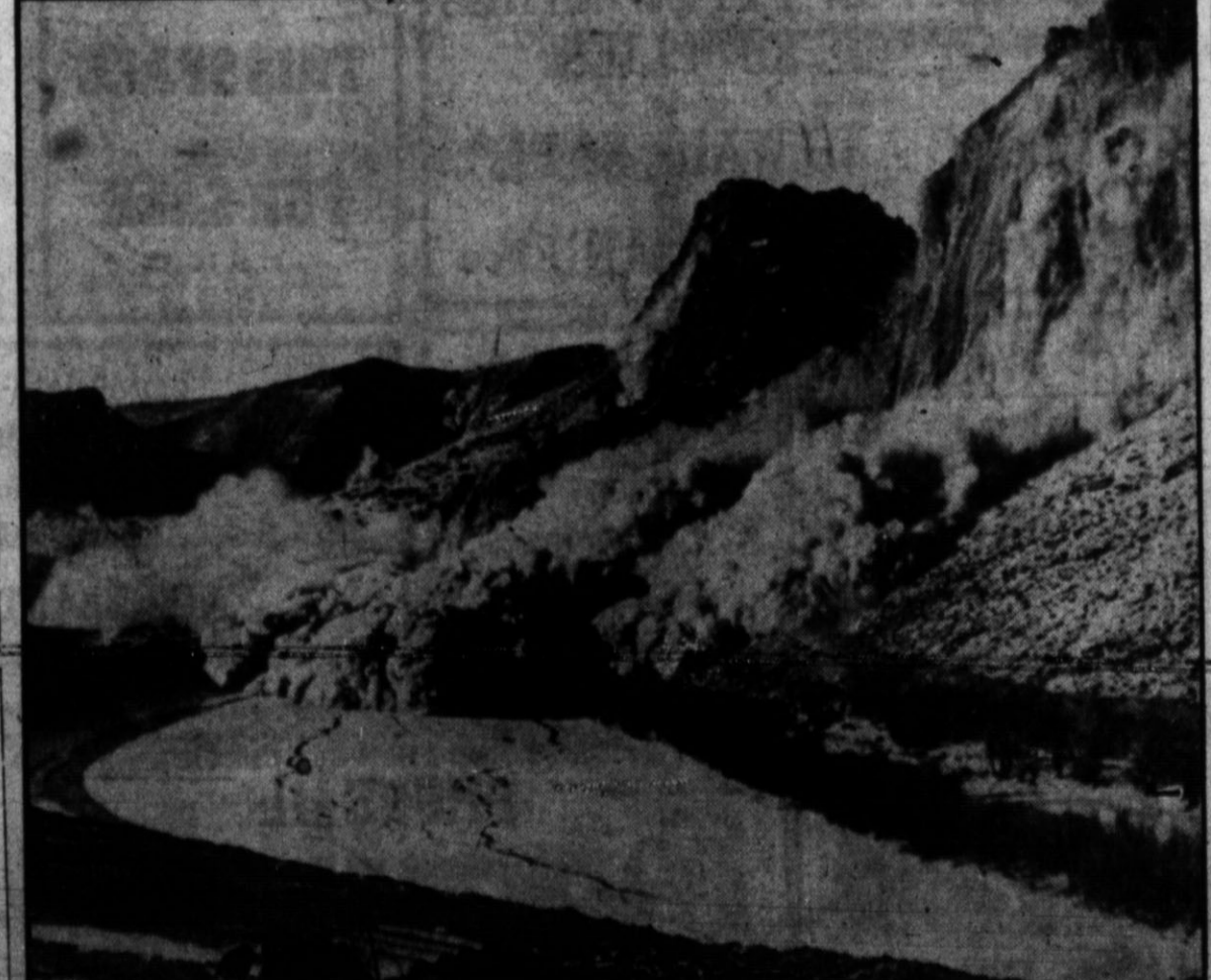
DYNAMITE BLASTS MOUNTAINSIDE —A mountainside erupts in this huge dynamite blast pictured at Boyan Dam, Wyo. More than 100 million pounds of rock were thrown loose by the 32 tons of dynamite used. Note the thick ice cracking in the Big Horn River at the mountain's base. An idea of the explosion's scale can be gained by noting the full-sized trees along the river bank.
