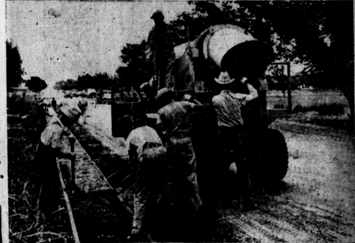
PAVING PROGRAM STARTS—As Hereford's $400,000 paving program started in July, above pictures were taken as workmen poured curb and gutter installations. As the program began, contractors estimated it would take from nine to 12 months to complete.
