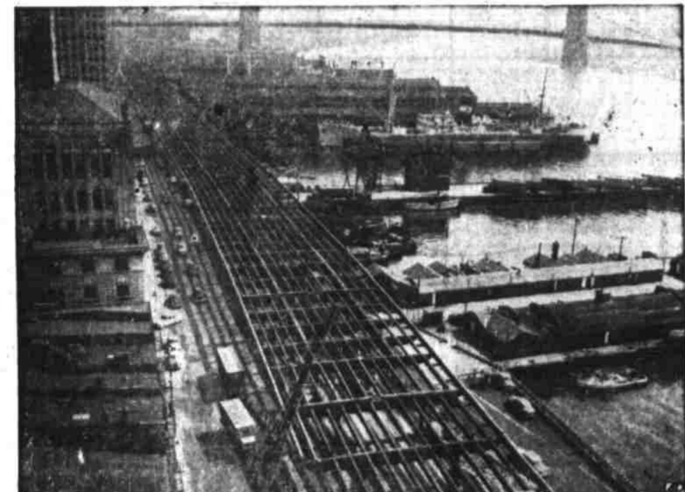
HIGHWAY SKELETON —Steel frame for stretch of elevated highway along New York's East River is completed. It will link with roads circling Manhattan's 24-mile perimeter.
