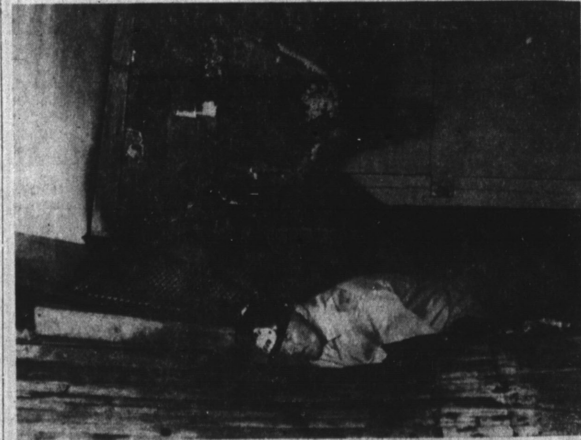
VOLUNTEER FIREMAN George Jowell helps extinguish flames under the floor of the high school industrial arts building Friday morning. Jowell is standing in a hole which was burned through the floor at the location of a gas floor furnace, where the fire started. Damage was estimated at about $2400 by Hereford Fire Marshal Clay Angelo. (Staff Photo)
