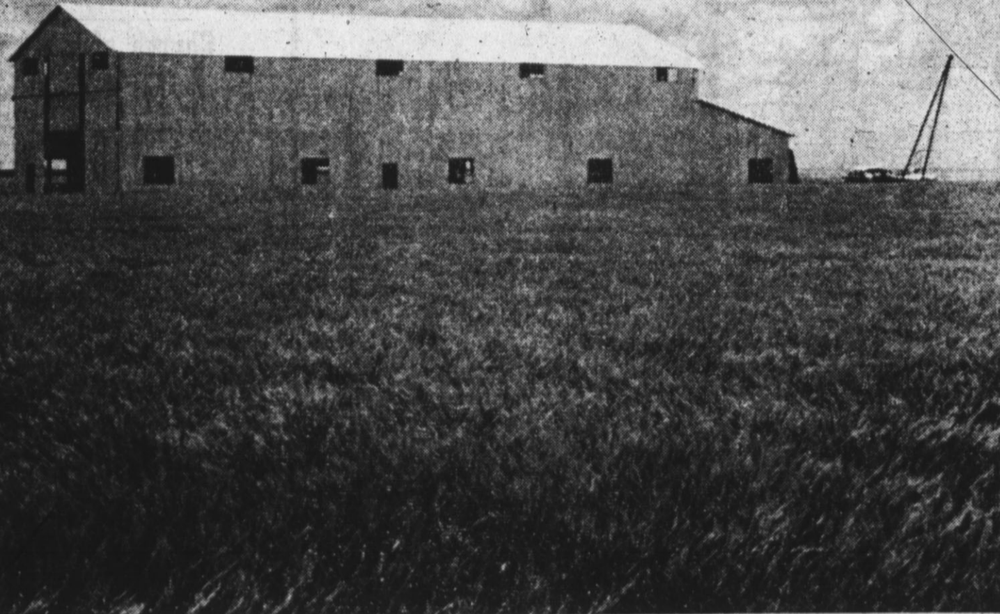
ALY COMPLETED—A new cotton gin presently under construction is nearing completion. The structure is being built due south of the Hereford Labor Camp. H. C. Barton of Lubbock is the owner. It will be the third cotton gin in Hereford. (Staff Photo)
