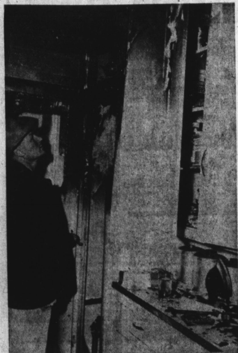
DAMAGE AT THE MUSE residence was given a thorough inspection early Tuesday morning by Hereford volunteer fireman Glen Nelson...
