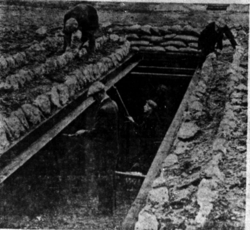
Workmen have completed one of the trenches dug on the grounds of the Imperial War museum in London during the war scare that preceded the Munich pact. Authorities will maintain the trenches as a permanent air-raid shelter in the event of future war. Safety measures of all kinds have been widely inaugurated throughout all of England as well as London.
