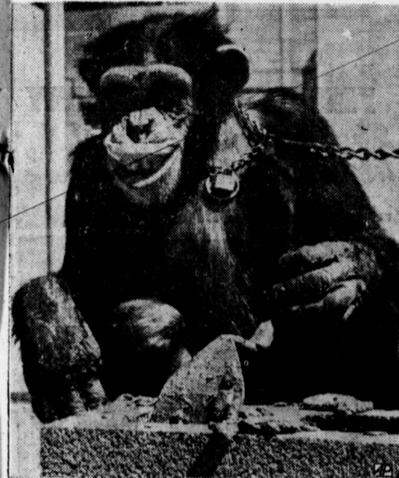
CONSTRUCTIVE CHIMP—Charlie the Chimp lends a hand and makes with the mortar as the new monkey house at Abilene's zoo nears completion. Charlie, an expert at many tricks, is a favorite with the children. (AP Wirephoto)
