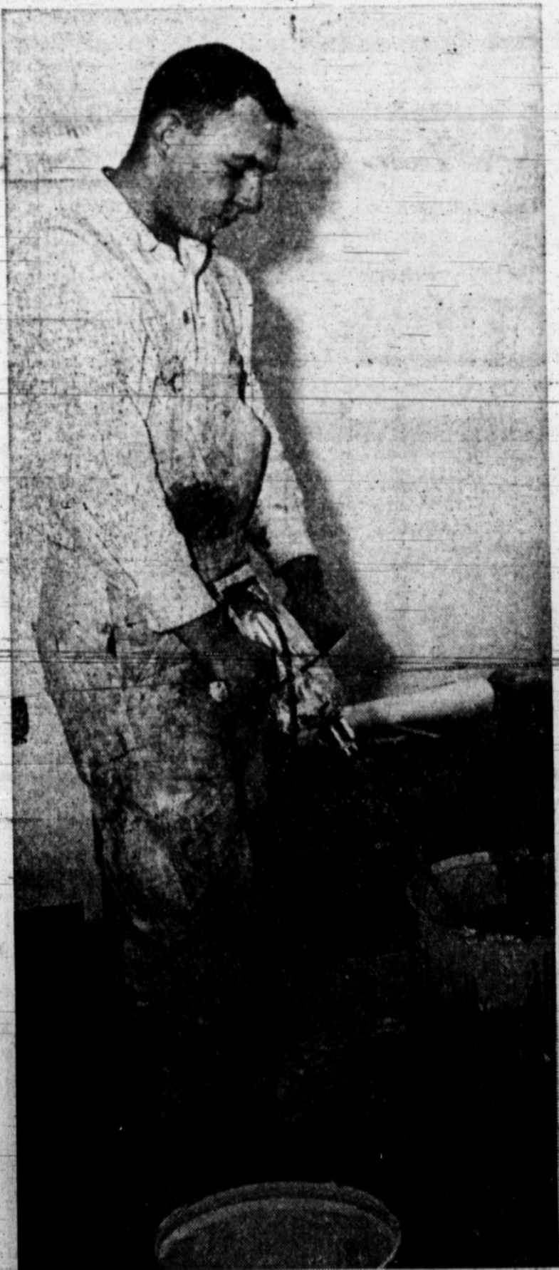
STIRRING SCENE —Charles Noland of Amarillo uses an electric mixer as he prepares paint for the new wing at the county hospital.
