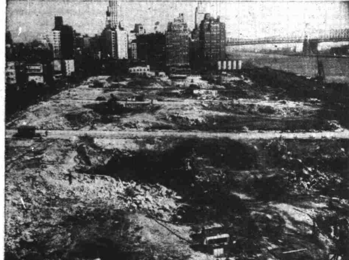
CLEAR U. N. SITE FOR CONSTRUCTION — This overhead view of the site of the permanent home of the United Nations on Manhattan's mid-town East Side, shows blasting crews, excavators and surveyors, clearing ground for construction.
