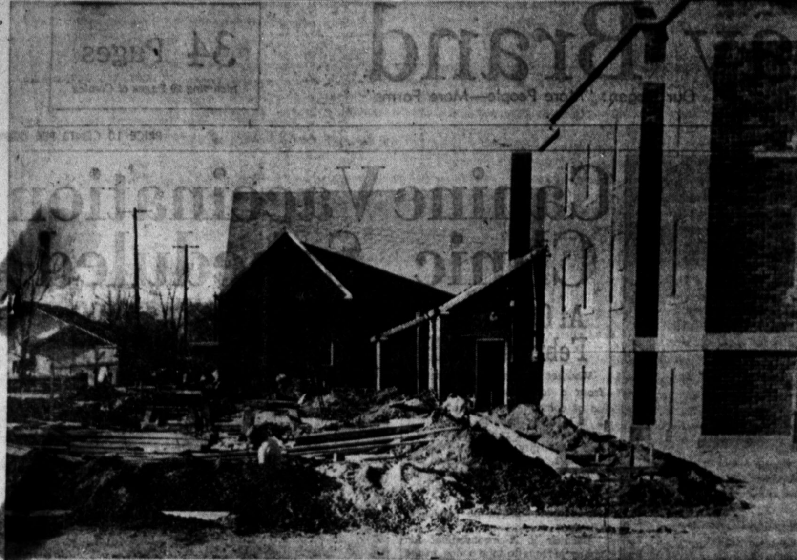
FOUNDATION WORK for the two-story educational building being erected by the First Methodist Church is well along. Work on the building may be completed with as little as 60 days, unless delays are caused by inclement weather, the contractor said before the work was begun. (Staff Photo.)
