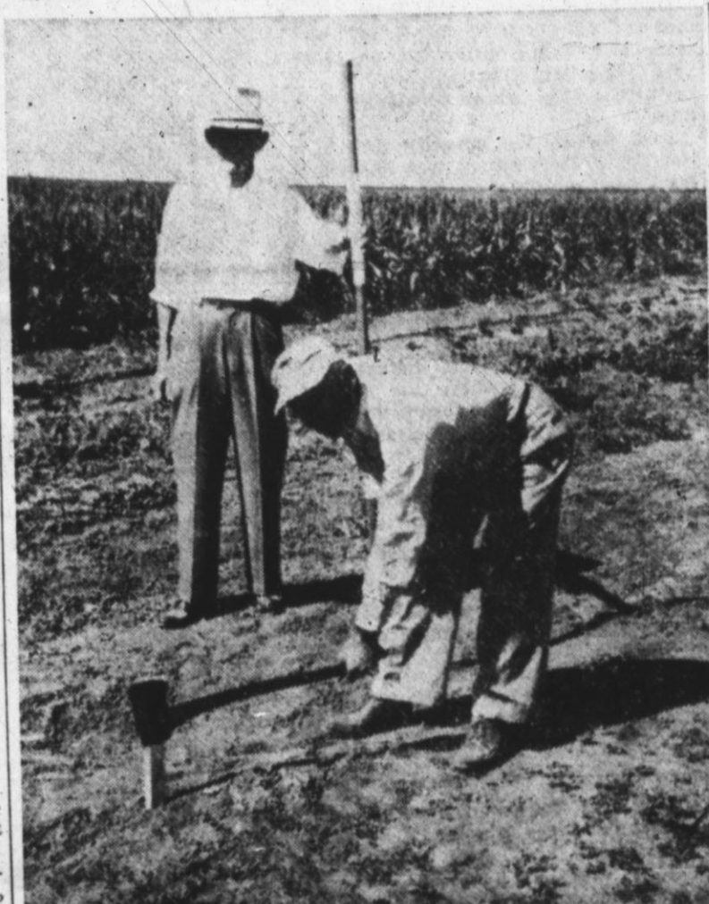
EDDIE REINAUER, president of the board of the West Texas Rural Telephone Cooperative, is shown driving the first stake for the 900-mile telephone network on the E. O. Billingslea farm northwest of Dawn. George Stambaugh is shown behind Reinauer holding a surveyor's measuring stick. Staff Photo.
