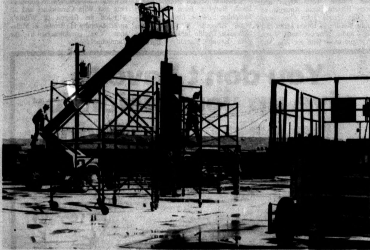
Work is underway on the first phase of the $625,000 expansion project at Hereford Senior Citizens Center. A $50,000 challenge grant has been awarded by the Mabee Foundation, and HSCA continues its fund raising for the project.
