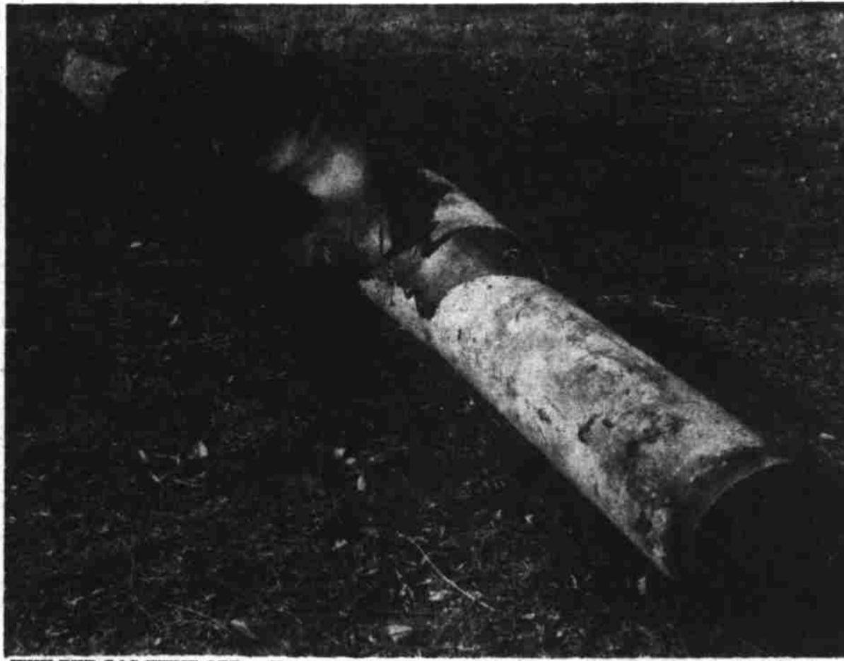
WHY THE GAS WENT OFF —Here's why the gas went off here a week ago Saturday. A 200-foot section of pipe, apparently in sound condition, shattered on the Empire Southern Gas company transmission line in Martin county, just west of the Howard county line. Gas, under 450 pounds of pressure from the Andrews production field, literally exploded the heavy pipe as it had been an ill-fated cannon barrel. The section, speedily replaced, was brought to the warehouse here. (Jack M. Haynes Photo).
