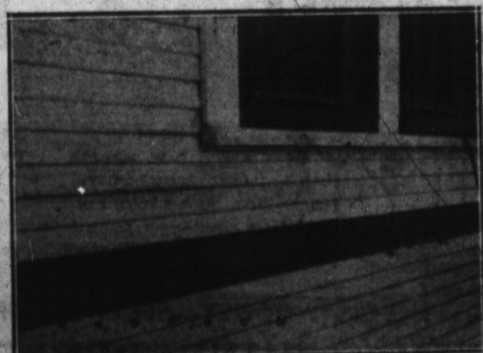
Side wall showing vacant space between up-rights and wall space filled with THERMAL WOOL
