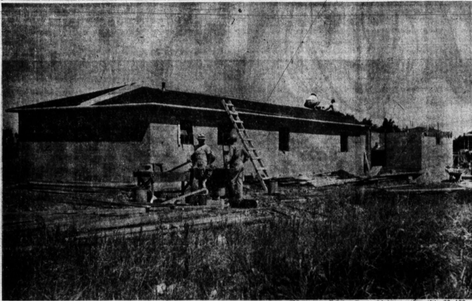
HERE IS WHAT ONE MAN IS doing to beat the direct housing shortage for migrant labor. John Paetzold is erecting this 20x130 concrete block dormitory to house from 30-50 workers on his company property on the west edge of the city. Labor is here now waiting to get into the dormitory, which will be finished next week. Besides the sleeping quarters, there is a large community kitchen, a dining room, and two big toilets and shower rooms. The dormitory will be "modern and sanitary in every respect", Paetzold said. The dormitory will house lettuce crews of Charlie Huston.
