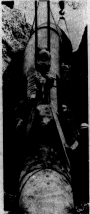
EASY DOES IT for a work crew lowering a section of the Alaska pipeline into a trench. Work on the line, which will run some 800 miles, alternately buried and elevated above the tundra from the North Slope oil fields to Port Valdez, continues despite leakage problems.
