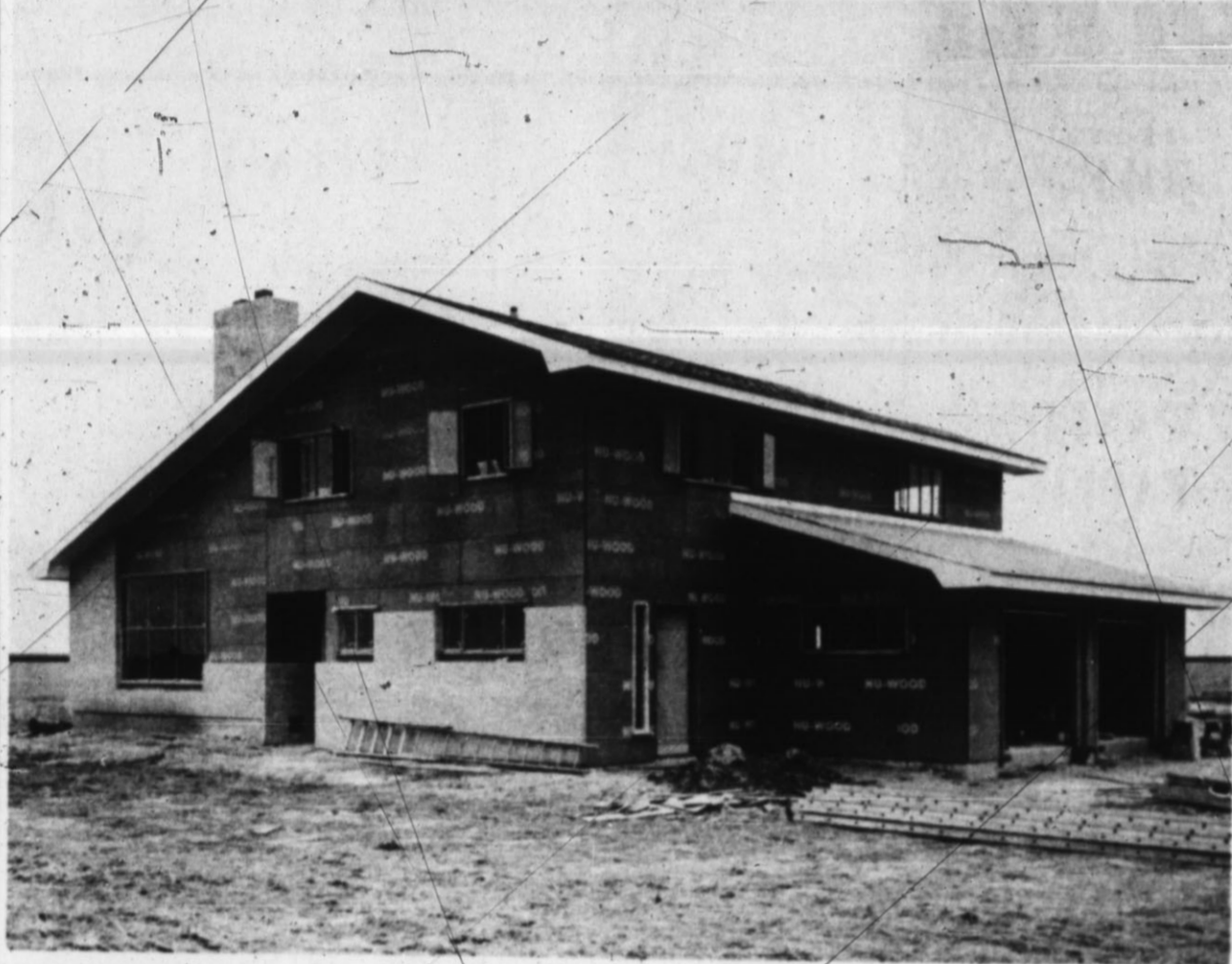
This Could Be Your Home Before . . . You Install Aluminum Siding
