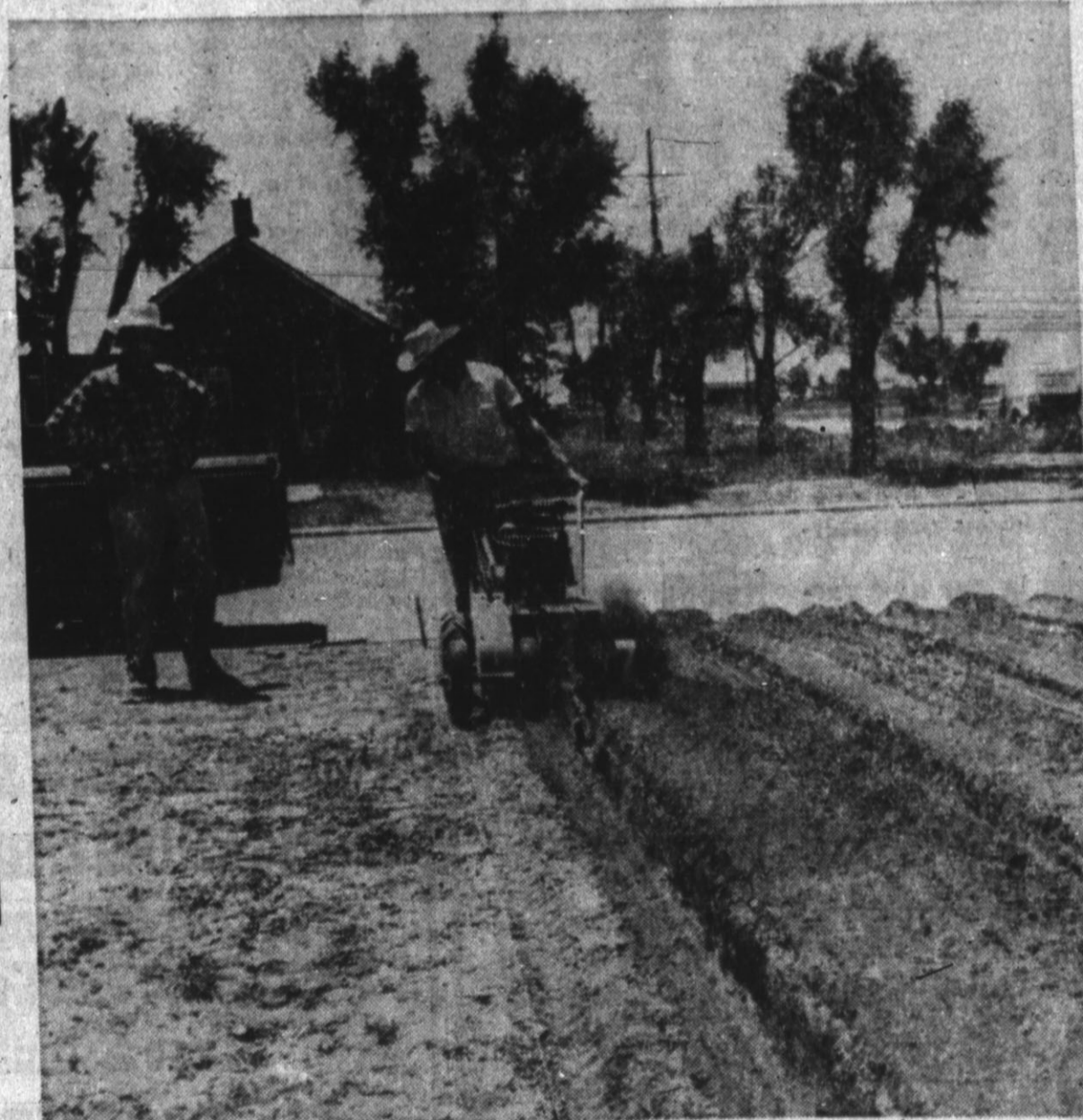
GEORGE SPRINGER is shown above operating the ditching machine during the installation of an underground system on a Hereford lawn. We invite you to Phone George at EM 4-1393 or one of the Bryant Bros. and let them give you an actual demonstration of the effectiveness of this new system.
