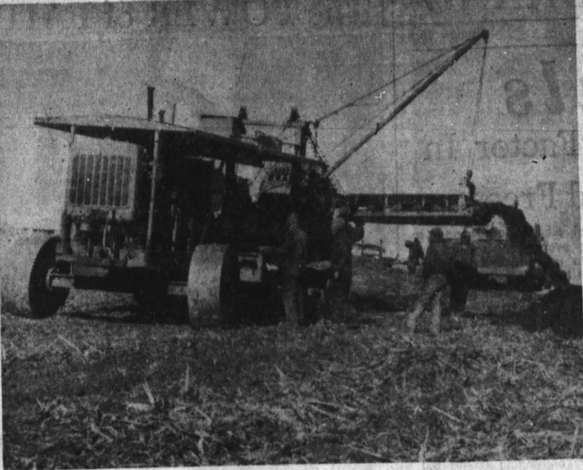
THROWING DIRT ASIDE, a huge ditcher Company of Houston is doing the work starts working on a 24-inch natural gas here for Transwestern Pipeline Company. (Staff Photo)
