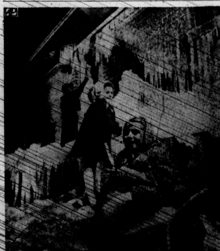
ICY NORTHER — The norther which struck across Texas left this broken pipe and icy house in Dallas. When expanding ice broke the pipe it sprayed water, which quickly froze, over the unoccupied house. (AP Wirephoto)
