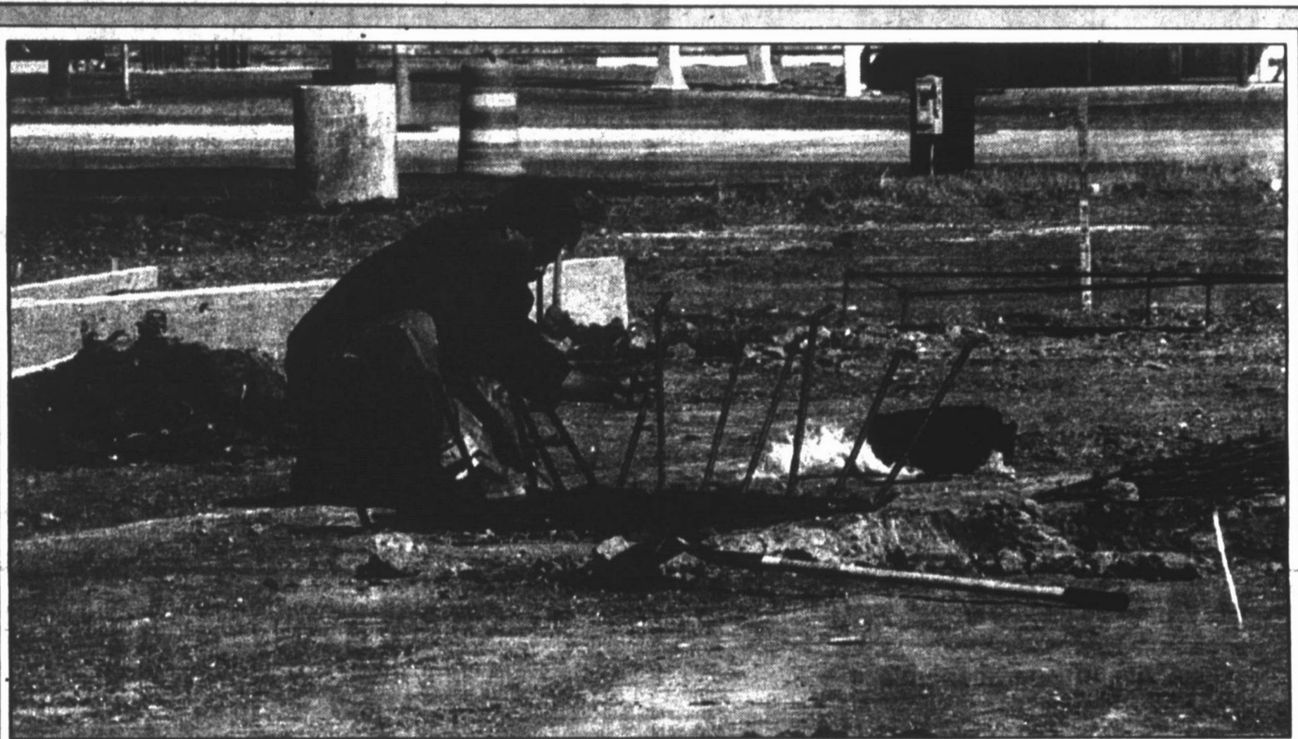
Preparing site — Tomas Lamas of Whiteface Concrete places reinforcement bars before the foundation is poured for Movie Video Gallery, which will be located in the 800 block of South 25 Mile Avenue. The 4,200-square-foot store is being built by GBH Development & Investment, a Texarkana, Ark.-based firm.
