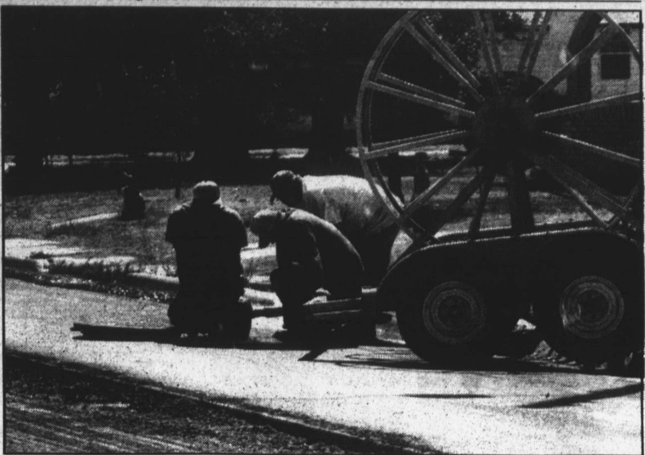
Getting it ready — The Mize brothers, (from left) Les, Bruce and Mark, pump water out of the sewer line in the 400 block of South 25 Mile Avenue, as they prepare to install fiber-optic telephone lines for Southwestern Bell Telephone Co. The Mizes operate Public Utilities Co. of Mobeetie.
