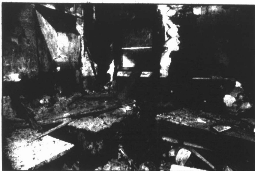
Proceeds from the sale of items (displayed at the Bull Barn, top) will be used to repair fire damage (above) and smoke damage (right) to a house which has been donated for use as a shelter.
