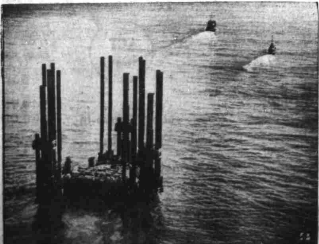
ON SCHEDULE — The 6,000-ton Texas-tower type "island" which will be offshore radar station in continental defense system is towed toward permanent location on George's Bank, 100-odd miles off the New England coast. Ocean-going tugs are Marion Moran, left, and M. Moran.
