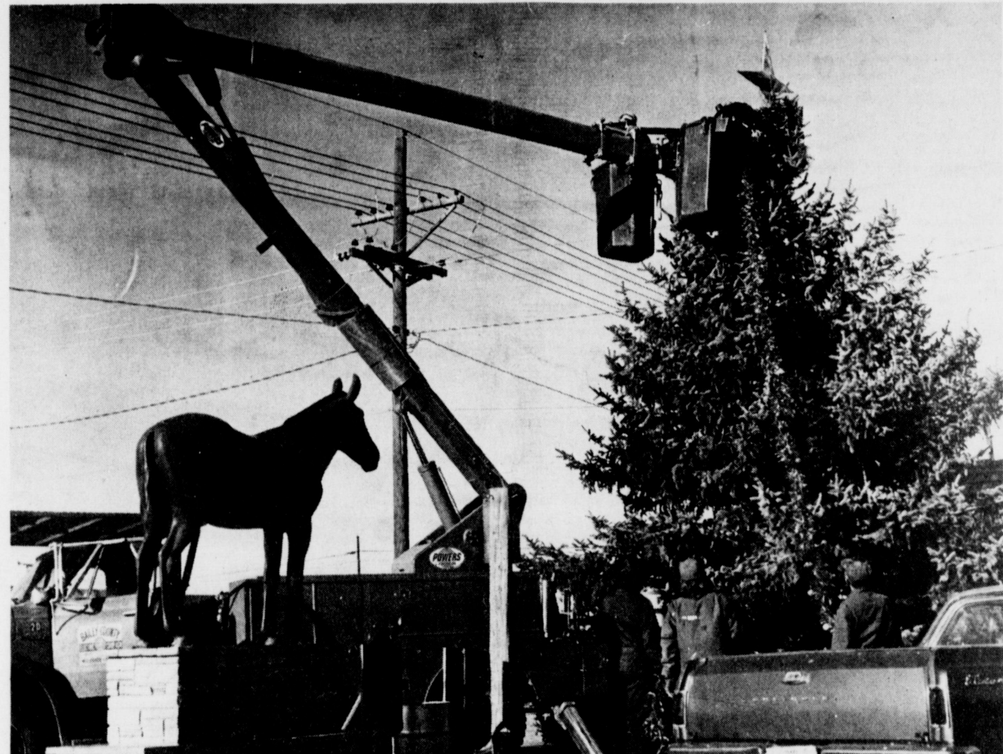
GETTING READY FOR CHRISTMAS . . . A huge Blue Spruce that once grew in the E.O. Baker yard, blew down during Saturday's wind storm but was salvaged and donated to the City of Muleshoe by the Bakers, for Christmas. Bailey County Electric put the tree up near the Mule Memorial and decorated it Thursday morning. Shown
