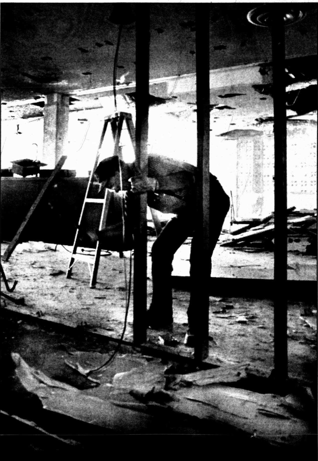
Bringing down the house -- Bank Design Construction Corporation out of Boerne, Texas will be here for three or four months refurbishing the former Energas building, at the corner of Third and Lee, into the new First National Bank of Hereford. Project manager Wayne Mitchell was captured knocking out the studs Wednesday as the remodeling got under way.
