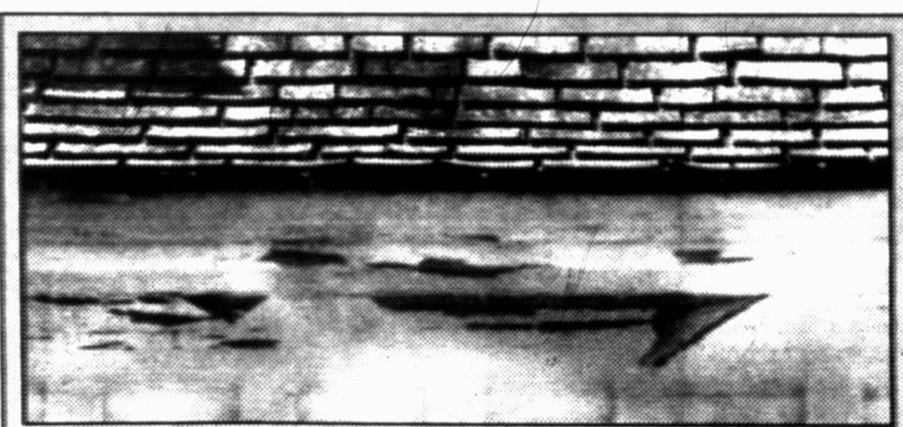
Paint is peeling away from under the eaves on the east side of the historic E.B. Black House.
