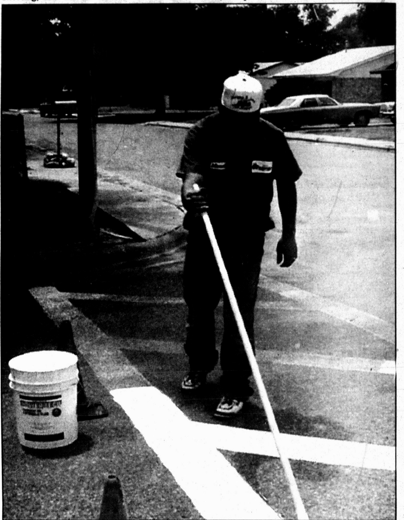
Prep work --- City streets worker Manuel Cantu began his back-to-school routine this week with the annual restriping of the crosswalks near the Hereford Independent School District campuses. School begins Aug. 16 for all campuses with teachers reporting as early as Aug. 9 for new teacher in-service and beginning day on Aug. 10. Teachers will spend the rest of next week in staff development.
