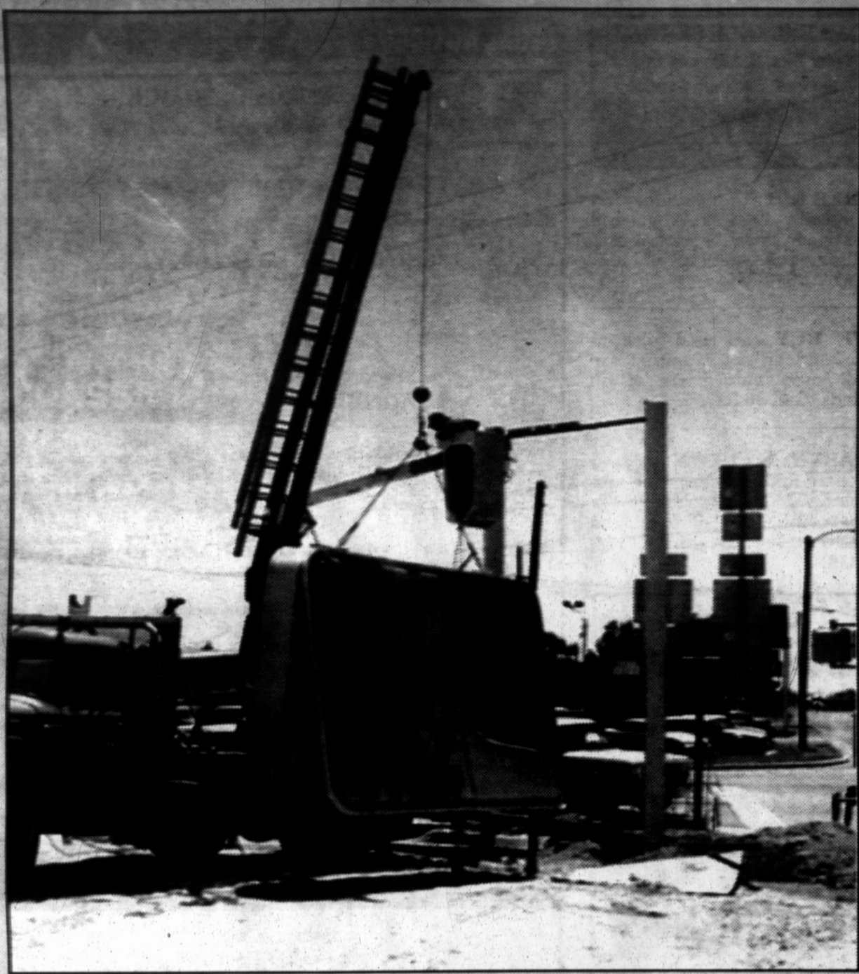
Sign almost ready — Workers for Hi-Plains Canvas Products of Amarillo were getting things ready Thursday for installation of the sign at the new Kentucky Fried Chicken restaurant near the intersection of South 25 Mile Avenue and U.S. Highway 60. Everything wasn't quite ready by the end of the work day, so the soon-to-open restaurant still didn't have its sign.
